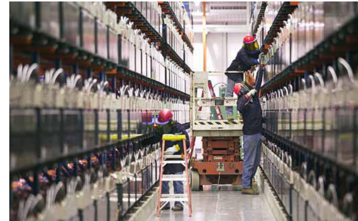
ABB Inc., Fairbanks, Alaska, 27 MW/15 minutes
