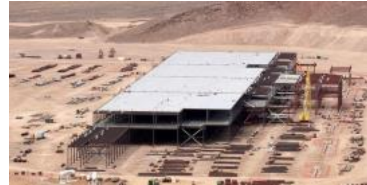
TESLA Plant, Nevada, Feb 2015
